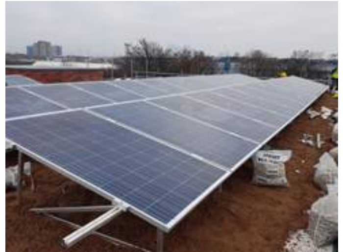
Green Roof and PV Panels
