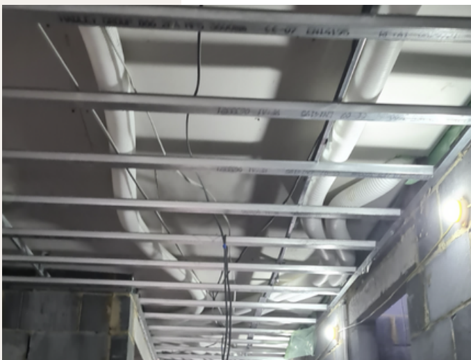
Ceiling & Ventilation Ducts
