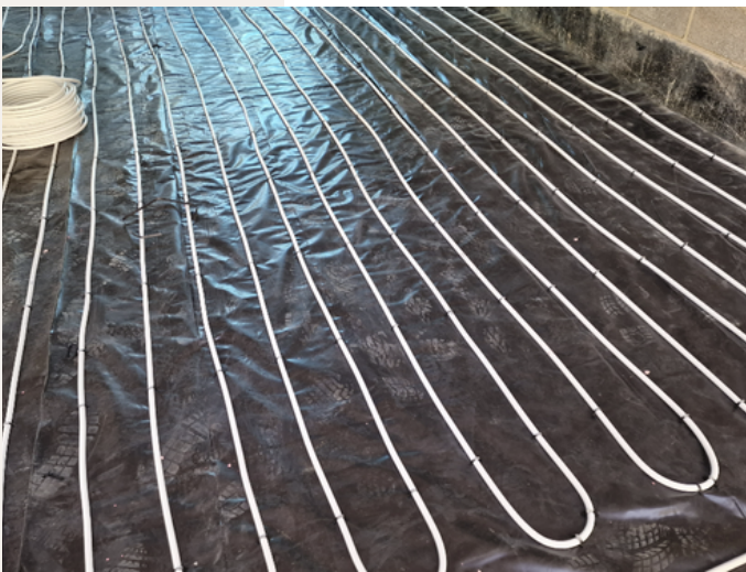
Under Floor Heating
